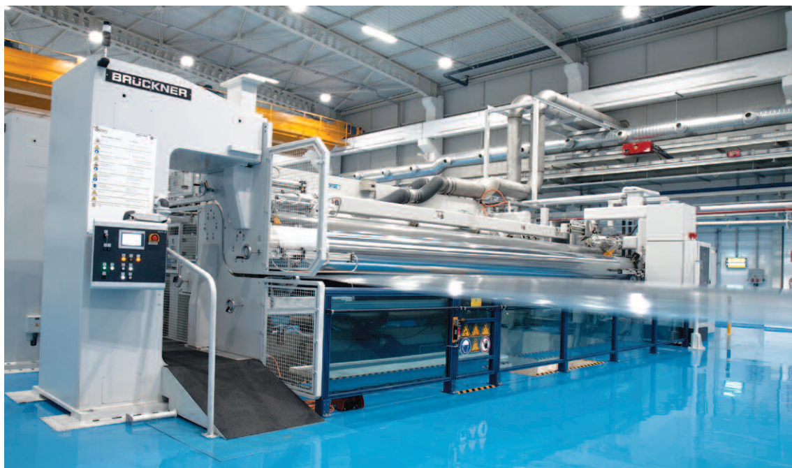
高效薄膜拉伸生产线 / Highly efficient film stretching line
